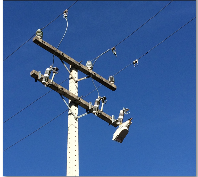
A TripSaver II recloser installation in Paraná, Brazil.
